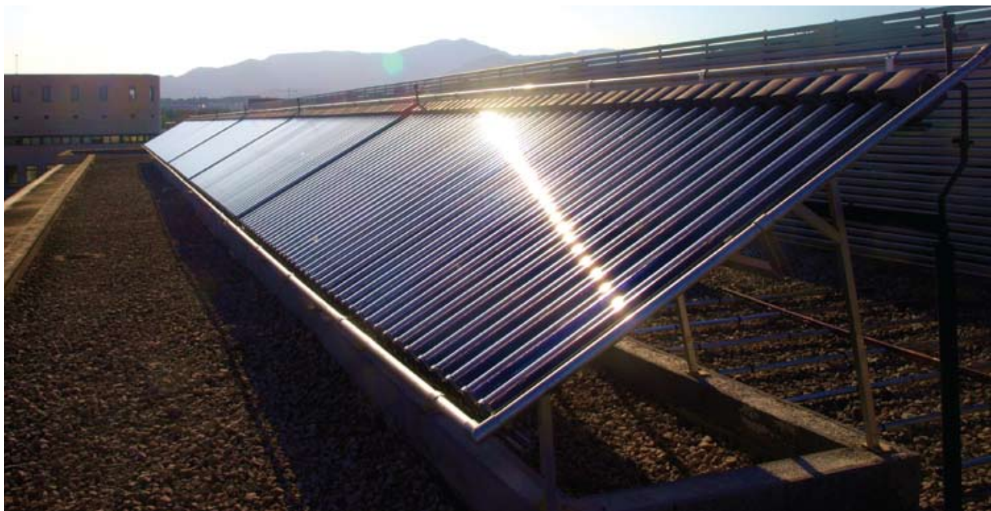
Solar hot water technology is currently a more mature technology than solar electric.
